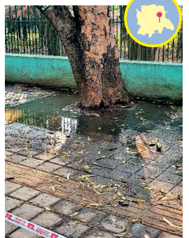
Water stagnation near Cubbon Park's new drain is causing a foul smell, which is noticeable even to travellers passing by.
